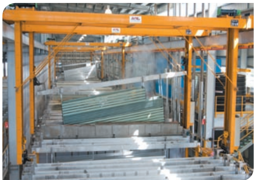
Anodising plant, Brisbane
